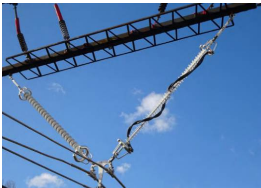
Short Circuit Test of 400kV suspension insulator string
