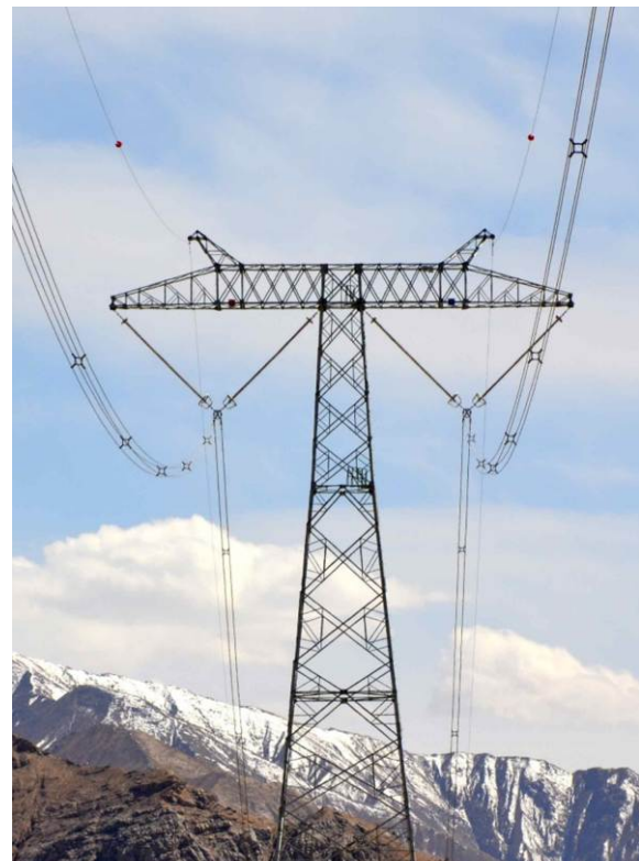
± 400kV DC Qinghai-Tibet Project
