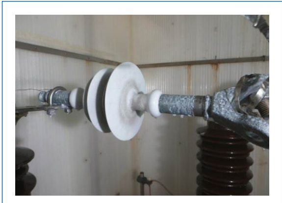
Tracking and Erosion Test (1000h salt fog method) of suspension insulator
