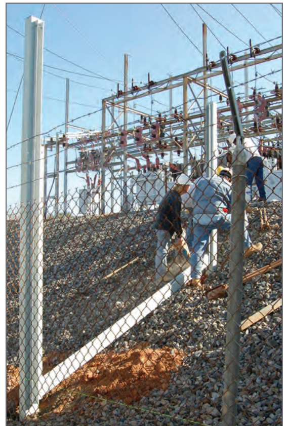
SafeFence is ideal for use on uneven terrain and can be easily modified during installation.
